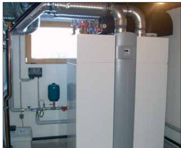
Figure 2. The integration of the air/water heat pump into the room ventilation controlled via KNX is the basis for the low energy demand
