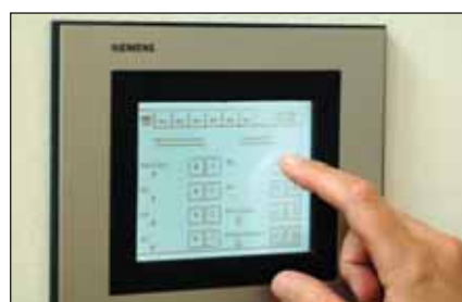
Figure 3. The operation of the building functions is performed through the touch panel UP 588 which is based on KNX RF.
