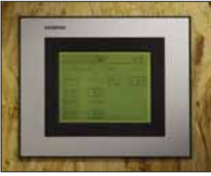
Fig. 4. The central control unit of the building control system is located in the mechanical room. Touch screens throughout the school allow access to all important functions.
