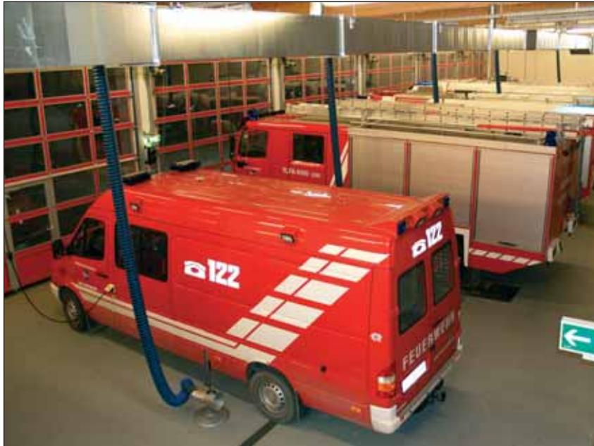
Picture 1. View into the vehicle hall of the new fire station in Obergrafendorf
