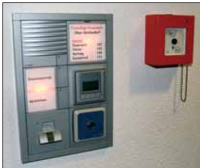
Picture 2. Thanks to the integration of different trades, the doors open and the lights are switched on by the fingerprint terminal of the access control system.
