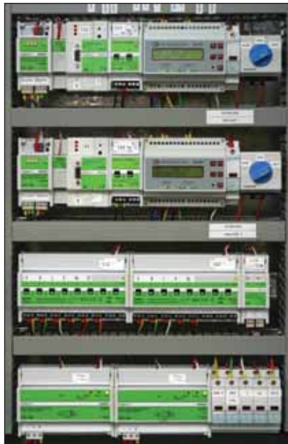
Picture 3: KNX components in the metering room of the attic.
