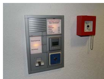
Figure 2. Thanks to the networking of the various trades, the doors are opened and the lights switched on via fingerprint access control. Source: HTL St Pölten
