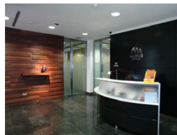
Figure 2 Via the KNX system access control interface (fingerprint), all facilities can be monitored and controlled as required. Source: ZVG
